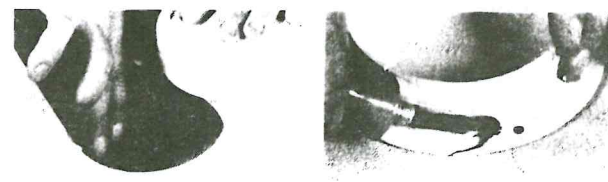
Sand the edges of the hole to insure a good fit and bed the deck ring with sealant. (NOTE: We used black sealant here for photographic purposes.)
